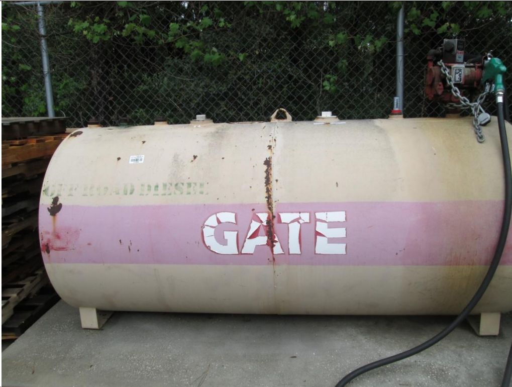
Photograph 17: Physical Plant, 500-Gallon Diesel AST
