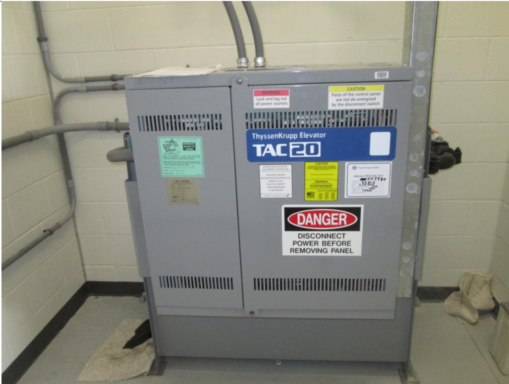
Photograph 10: MSRI, 60 Gallon Reservoir Hydraulic Elevator
