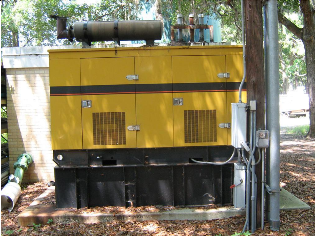
Photograph 22: Water Treatment Plant, Emergency Generator
