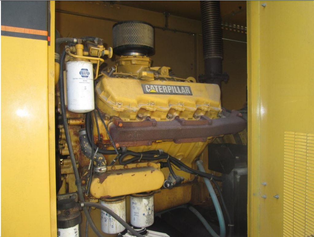
Photograph 23: Water Treatment Plant, 100 Gallon Diesel Emergency Generator
