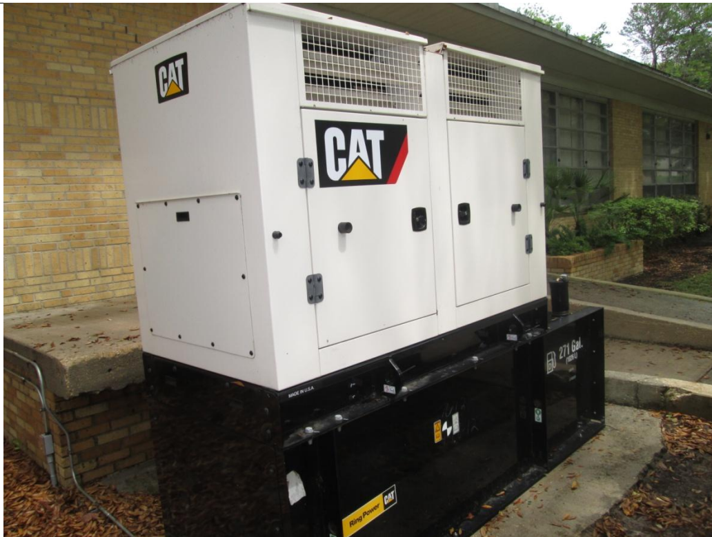
Photograph 4: Founders Hall, 271 Gallon Diesel Emergency Generator
