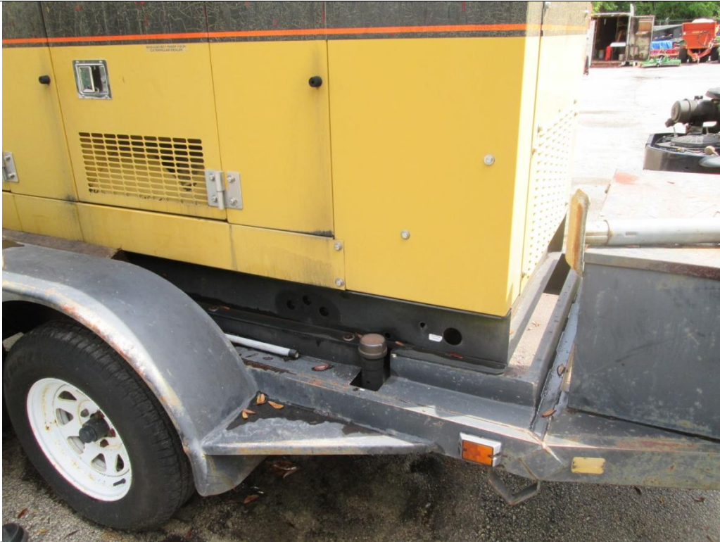
Photograph 15: Physical Plant, 60 Gallon Diesel Emergency Generator
