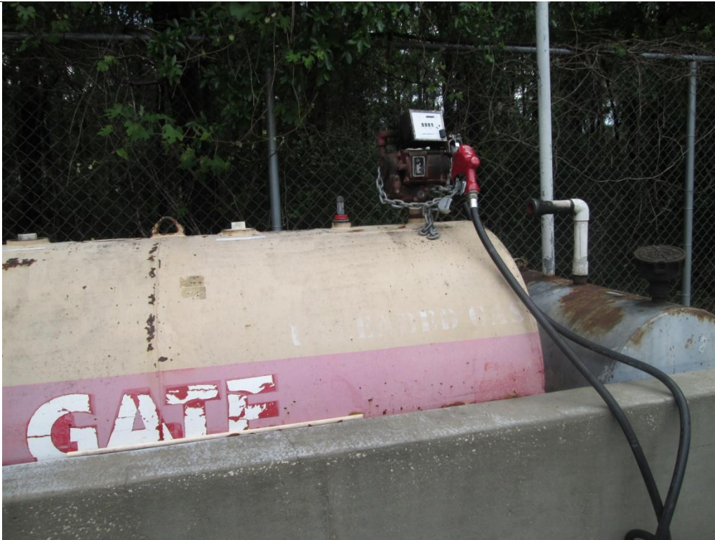
Photograph 18: Physical Plant, 500 Gallon Gasoline AST
