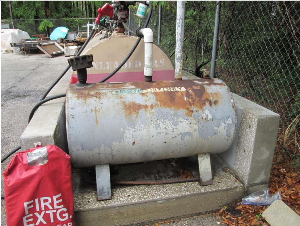
Photograph 16: Physical Plant, 250 Gallon Used Oil AST
