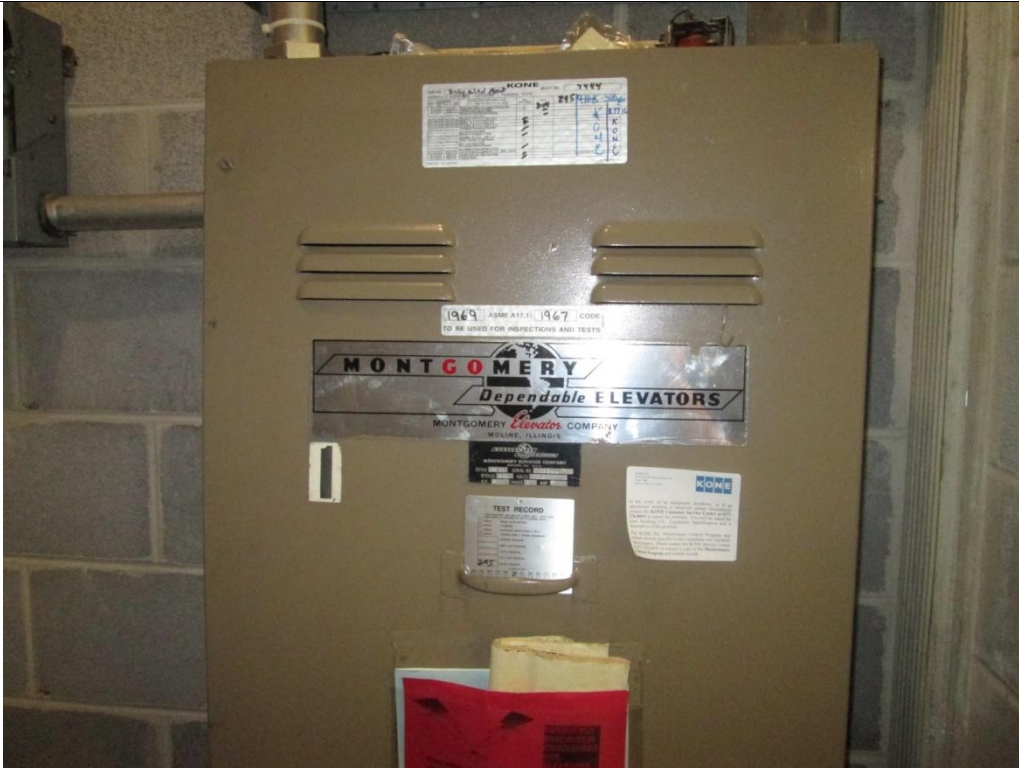
Photograph 21: Swisher Library, 100-Gallon Reservoir Hydraulic Elevator
