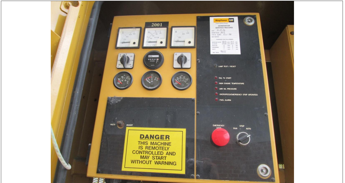
Photograph 11: MSRI, 382 Gallon Diesel Emergency Generator
