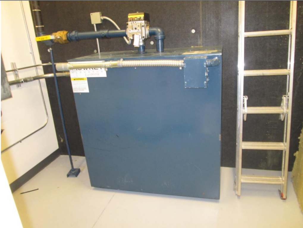
Photograph 1: College of Health Science, 132 Gallon Reservoir Hydraulic Elevator
